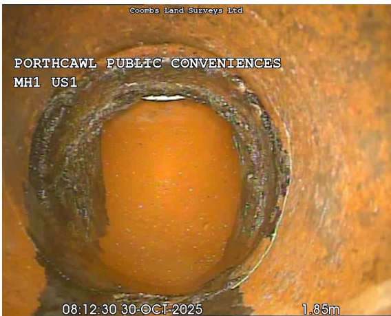
MH1US1X_35d39d28-a6a5-4248-b4f1-657a1669a3c3_20251030_135424_152.jpg, 00:00:26, 1.85 m Crack, circumferential at joint from 2 o'clock to 9 o'clock
