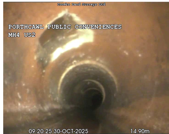
MH4US2X_37c44d2c-2031-455a-8325-96fc91747aee_20251031_092008_466.jpg, 00:01:36, 14.77 m Connection other than junction at 11 o'clock, 100mm dia
