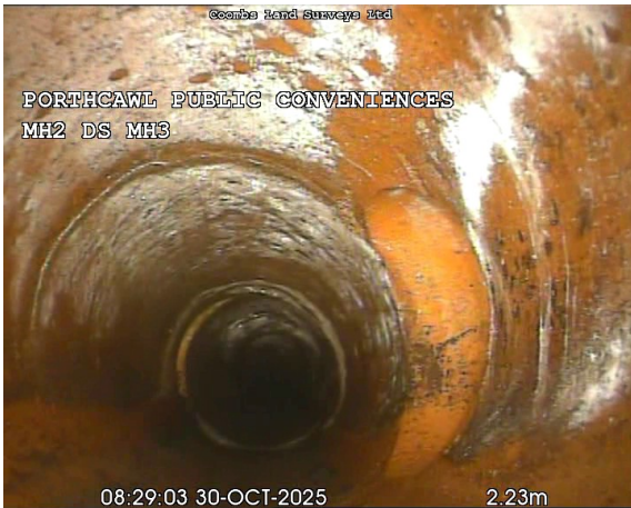
MH2X_dba9821f-c952-4f46-9e11-0361ac2a3d84_20251030_153017_552.jpg, 00:01:14, 2.23 m Crack, circumferential from 9 o'clock to 2 o'clock
