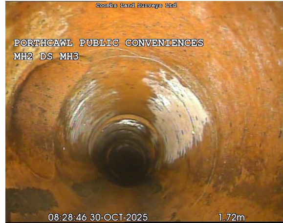
MH2X_af545427-5afb-4e4b-8427-72e837887416_20251030_152302_762.jpg, 00:00:57, 1.72 m Junction at 10 o'clock, 100mm dia
