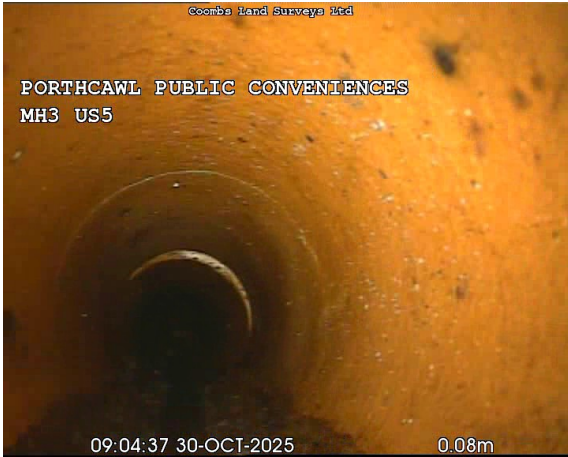
MH3US5X_462c77bc-30c1-4a98-b1bd-36cdeedc973d_20251 030_160336_884.jpg, 00:00:03, 0.20 m Crack, circumferential from 9 o'clock to 3 o'clock
