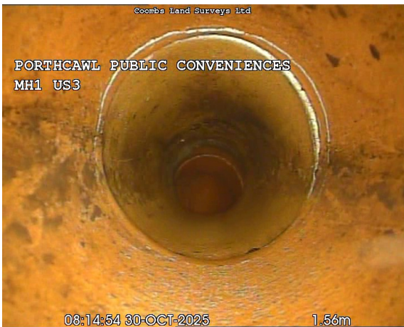
MH1US3X_18aabc77-7de4-4c1f-af0f-1b07af7aeefc_20251030_141937_026.jpg, 00:00:27, 1.56 m Crack, circumferential at joint from 9 o'clock to 4 o'clock
