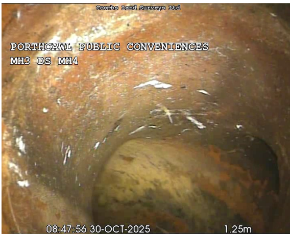
MH3X_b4968c10-8173-4a80-bf40-56862db04f1b_20251030_161739_248.jpg, 00:00:28, 1.25 m Junction at 3 o'clock, 100mm dia, Possible junction, angle not visible
