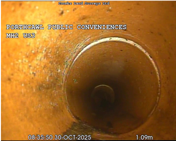
MH2US3X_89e84666-b551-404f-8aa7-d303a931c3de_20251030_150435_681.jpg, 00:00:08, 1.09 m Crack, circumferential at joint from 9 o'clock to 2 o'clock
