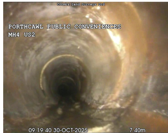
MH4US2X_a3898dd6-da3d-4d50-812a-dec2928405b5_20251031_091650_360.jpg, 00:00:52, 7.40 m Crack, circumferential from 7 o'clock to 5 o'clock
