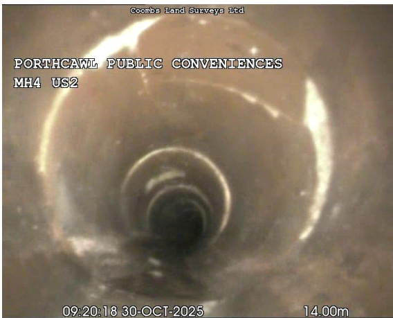
MH4US2X_5001f75c-b014-46ec-9a17-83cf11271024_20251031_091920_851.jpg, 00:01:30, 14.00 m Cracks, multiple at joint from 11 o'clock to 3 o'clock
