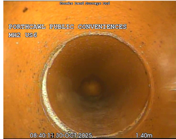
MH2US6X_da967db4-977d-42e5-b4fc-c4efc44c95ee_20251030_151539_701.jpg, 00:00:40, 1.40 m Crack, circumferential at joint from 2 o'clock to 11 o'clock
