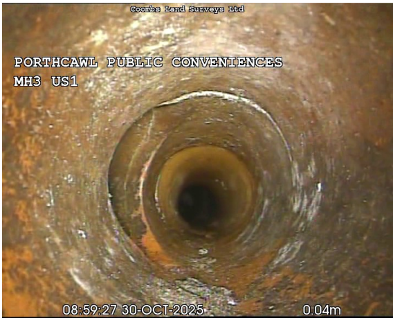
MH3US1X_74de2e3a-2ff8-42c5-b4c9-5148ae7bae50_20251030_154937_906.jpg, 00:00:04, 0.20 m Fracture, circumferential from 11 o'clock to 3 o'clock
