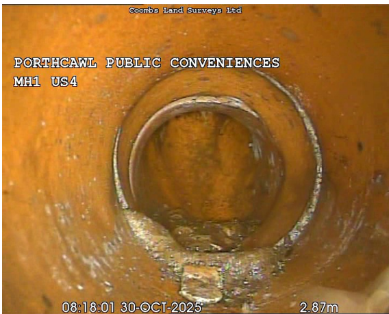
MH1US4X_1e7e6131-fb4d-4a00-9db6-0230afe08020_20251030_142839_440.jpg, 00:00:55, 2.87 m Attached deposits, fouling at joint from 5 o'clock to 8 o'clock, 10% cross-sectional area loss
