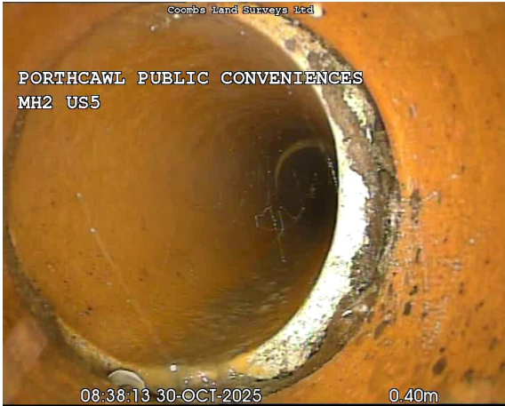
MH2US5X_044a7ba0-7c0d-473e-b719-53afab3cb3c7_20251 030_151028_344.jpg, 00:00:11, 0.40 m Joint displaced, medium
