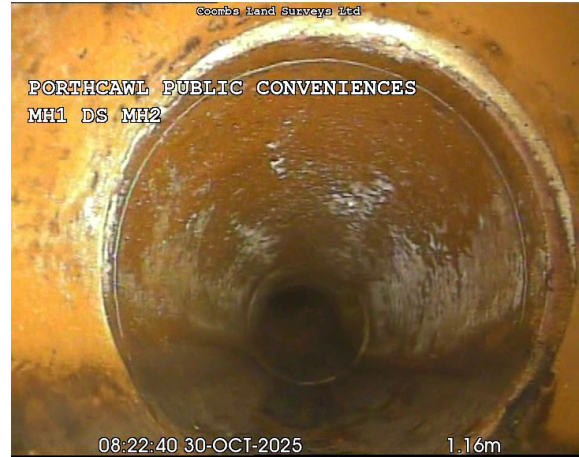
MH1X_d6316030-9abc-430a-a546-3e3af8964508_20251030_143422_601.jpg, 00:00:18, 1.16 m Crack, circumferential at joint from 9 o'clock to 3 o'clock
