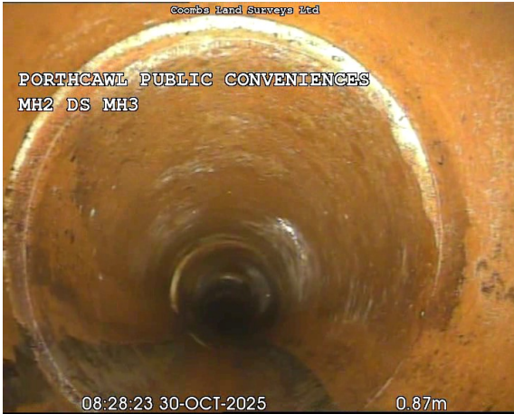
MH2X_fbfb30b6-0317-43e1-89d0-3bdf7efc708d_20251030_152116_464.jpg, 00:00:34, 0.87 m Crack, circumferential at joint from 3 o'clock to 1 o'clock
