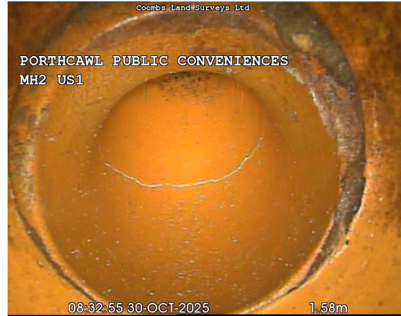
MH2US1X_f1b127c7-808b-45a2-bdb2-fd78384adb0e_20251030_144000_851.jpg, 00:00:40, 2.00 m Crack, circumferential from 3 o'clock to 9 o'clock, Crack in soil pipe bend
