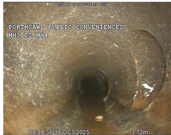
MH3X_290f36a5-6c77-42d8-b27b-cc6f493bf65a_20251030_162455_190.jpg, 00:01:23, 3.64 m Junction at 3 o'clock, 100mm dia
