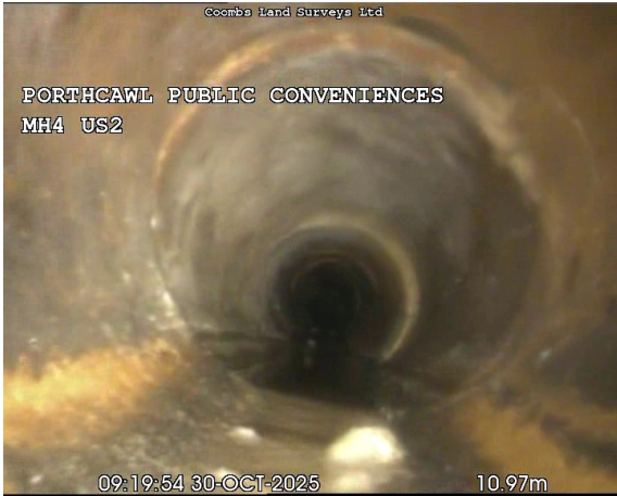
MH4US2X_ee0d96a3-61f4-4664-8a7f-cfd22c26969d_20251031_091751_040.jpg, 00:01:06, 10.97 m Hole in drain or sewer at 1 o'clock
