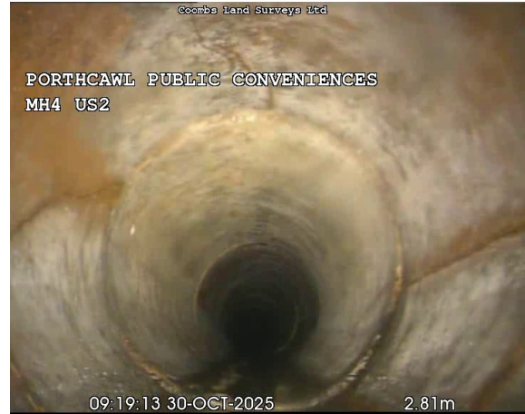
MH4US2X_76ce77ee-adeb-47fb-8121-9e37b45ba4fd_20251031_090701_052.jpg, 00:00:24, 2.81 m Crack, longitudinal at joint at 9 o'clock
