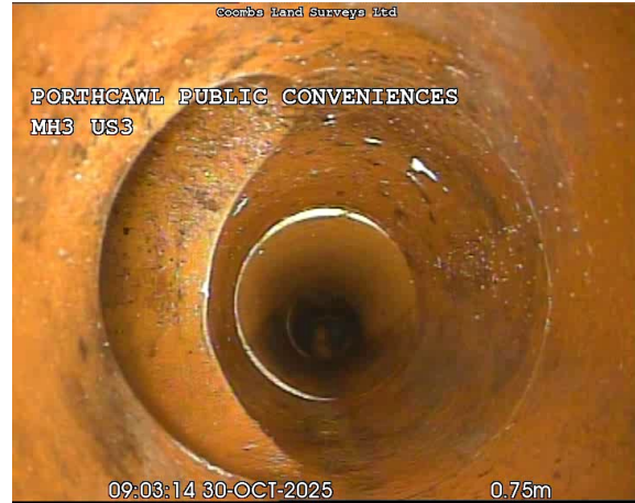
MH3US3X_e4f246da-fd53-46d9-bf61-c72d68cffbd9_20251030_160012_152.jpg, 00:00:07, 0.75 m Crack, circumferential from 11 o'clock to 6 o'clock
