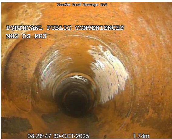
MH2X_b2e7adbb-e48d-4bf4-a58c-0502e74da5db_20251030_152841_927.jpg, 00:00:58, 1.74 m Crack, circumferential from 11 o'clock to 5 o'clock
