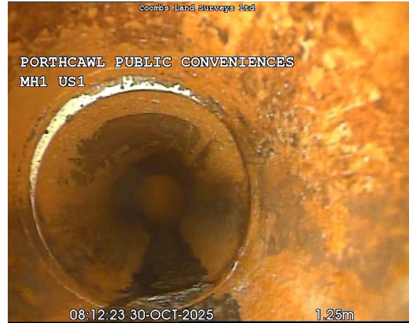
MH1US1X_bb479cf7-1870-4736-a41d-ca543cdf48cf_20251030_135346_717.jpg, 00:00:19, 1.25 m Crack, circumferential at joint from 4 o'clock to 1 o'clock
