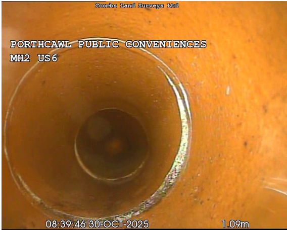
MH2US6X_b112e3bf-49e3-4884-bfa3-28048fc7a24f_20251030_151446_794.jpg, 00:00:14, 1.09 m Crack, circumferential at joint from 12 o'clock to 12 o'clock
