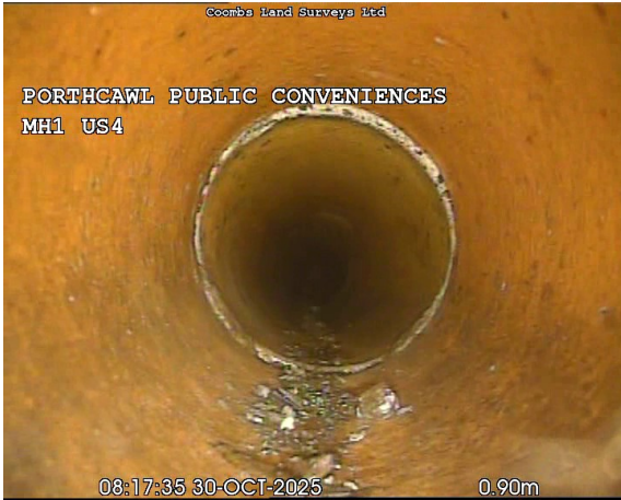
MH1US4X_a373b7c8-df1f-44d8-8cdb-fbb5e3582b5e_20251030_142704_142.jpg, 00:00:28, 0.90 m Settled deposits, coarse, 5% cross-sectional area loss, start
