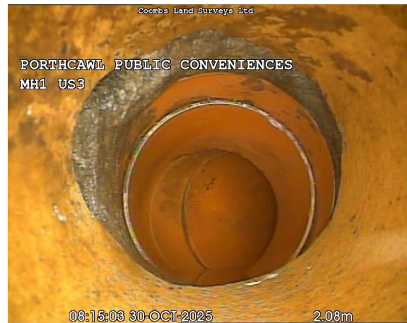
MH1US3X_f84c4ec4-59da-4a26-b49e-df870da98231_20251030_142026_593.jpg, 00:00:36, 2.08 m Point repair, pipe replaced from 12 o'clock to 12 o'clock, New pipe displaced but not open
