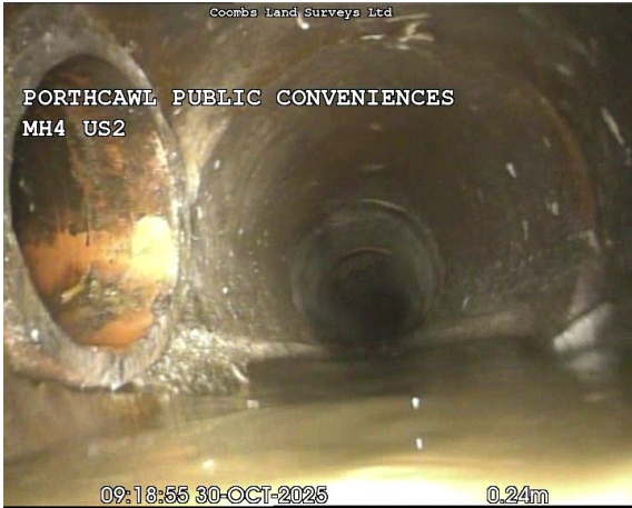
MH4US2X_ff93dd20-3959-4258-8813-d242b4256182_20251031_090608_715.jpg, 00:00:07, 0.24 m Connection other than junction at 9 o'clock, 150mm dia, from MH3, Incoming connection from MH3
