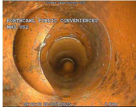
MH3US2X_6fcf7c1a-bb80-43db-8e49-3b5e8115a976_20251030_155627_672.jpg, 00:00:14, 0.89 m Crack, circumferential from 11 o'clock to 6 o'clock
