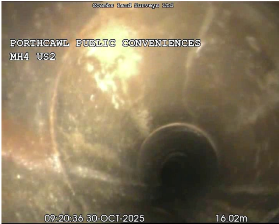
MH4US2X_8f7ae233-c6f9-4b44-b1de-da72e3b17c72_20251031_092104_735.jpg, 00:01:47, 16.02 m Crack, longitudinal at 12 o'clock
