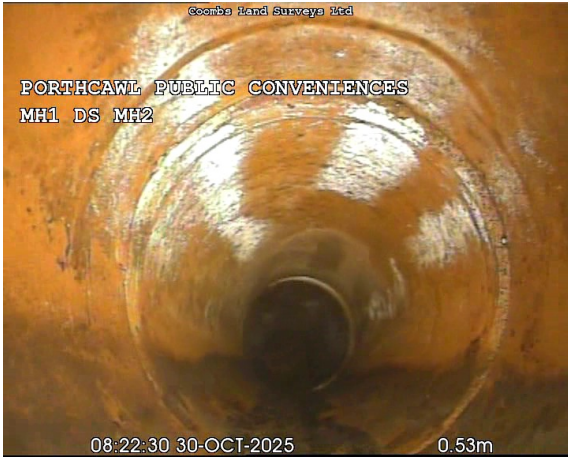
MH1X_64b42b8e-8778-4ea4-a00d-7cb4edd1c734_20251030_143350_153.jpg, 00:00:08, 0.53 m Crack, circumferential at joint from 9 o'clock to 3 o'clock
