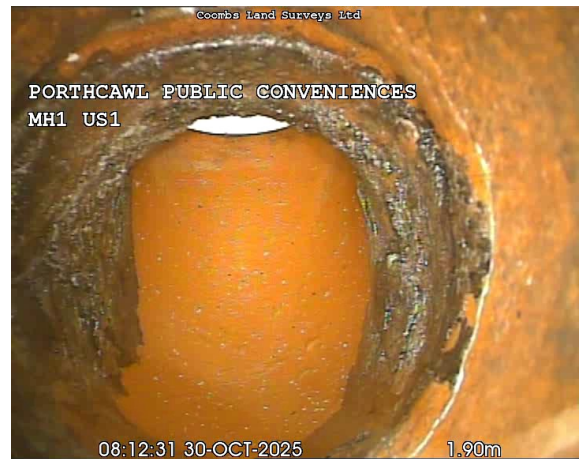
MH1US1X_39bca0f4-511e-4277-969b-f1764c5d47cf_20251030_140113_004.jpg, 00:00:28, 1.90 m Attached deposits, fouling from 12 o'clock to 12 o'clock, 5% cross-sectional area loss
