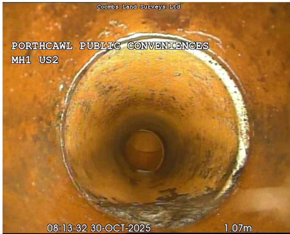
MH1US2X_ab9f18e7-a0e0-4689-b1db-4f3869930562_20251030_141103_704.jpg, 00:00:26, 1.07 m Crack, circumferential at joint from 7 o'clock to 2 o'clock
