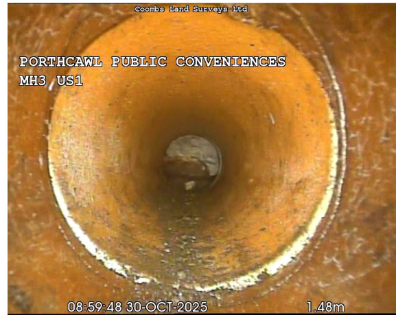
MH3US1X_bfcb32a5-432b-4533-b03e-1a2966a8b1a5_20251030_155128_573.jpg, 00:00:25, 1.48 m Crack, circumferential at joint from 12 o'clock to 8 o'clock
