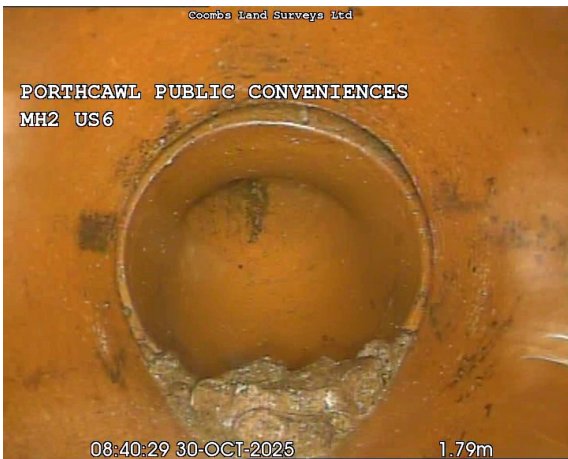
MH2US6X_23205f73-e479-4c4f-8782-7ee589f2acb6_20251030_151621_022.jpg, 00:00:58, 1.80 m Attached deposits, fouling at joint from 5 o'clock to 7 o'clock, 15% cross-sectional area loss
