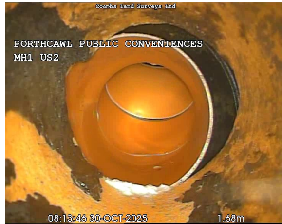
MH1US2X_0ad361e2-f698-4d57-a495-2d819d79bd3d_20251030_141315_944.jpg, 00:00:39, 1.68 m Point repair, pipe replaced from 12 o'clock to 12 o'clock, New pipe displaced but not open
