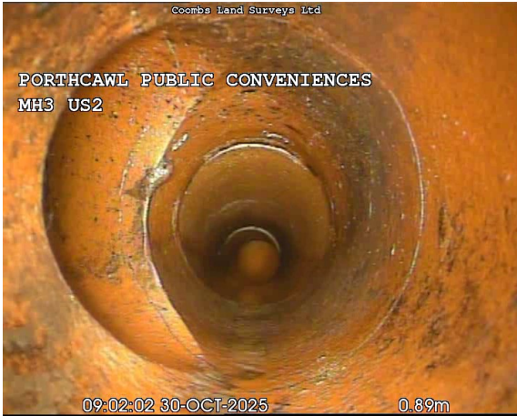
MH3US2X_9ded3e5a-d1b2-4c25-bc98-1abae4747150_20251030_155613_235.jpg, 00:00:14, 0.89 m Junction at 9 o'clock, 100mm dia
