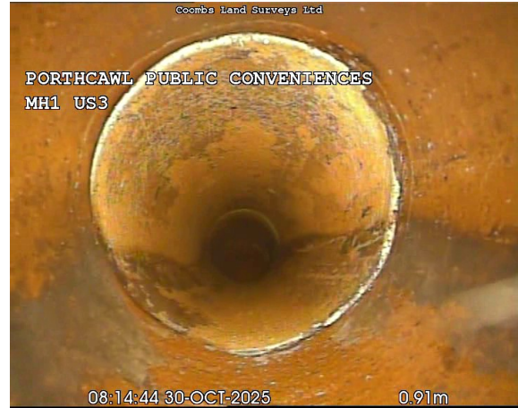
MH1US3X_7055dc70-6695-46ab-b64e-ebad8ac8fc5d_20251030_141848_545.jpg, 00:00:17, 0.90 m Crack, circumferential at joint from 9 o'clock to 3 o'clock
