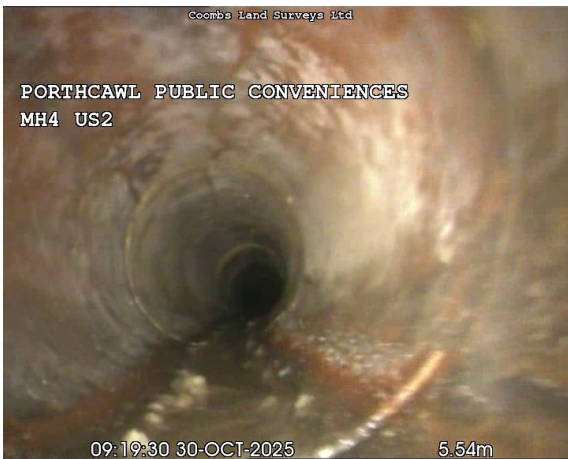
MH4US2X_31183ad8-1d3a-4356-8b02-1c927edcfb64_20251031_091614_018.jpg, 00:00:41, 5.54 m Crack, longitudinal at joint at 12 o'clock
