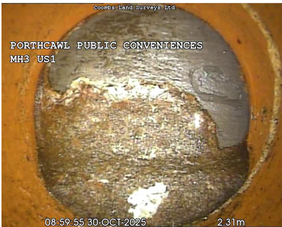
MH3US1X_eac89e69-8f42-4753-b16f-297848715ff8_20251030_155246_683.jpg, 00:00:33, 2.39 m Finish node, other special chamber, reference: MH3US1, Pipe capped off
